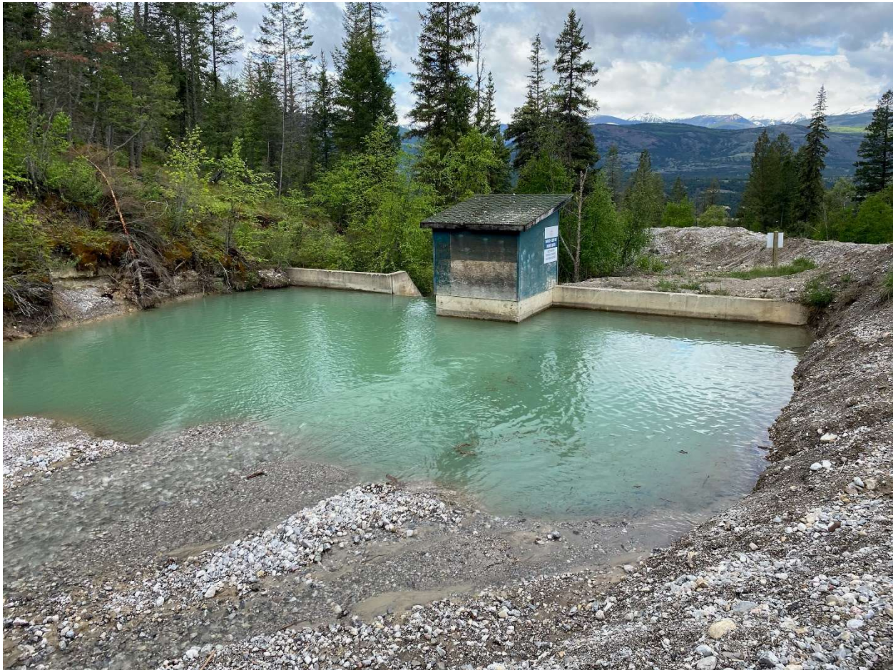
Photo 1: Cold Spring Creek Dam Reservoir approximately 75% filled with debris. May 28, 2021.
