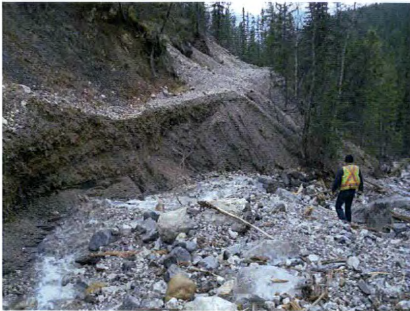
Washed out cross-country ski trail along north tributary (Oct. 15, 2012)
