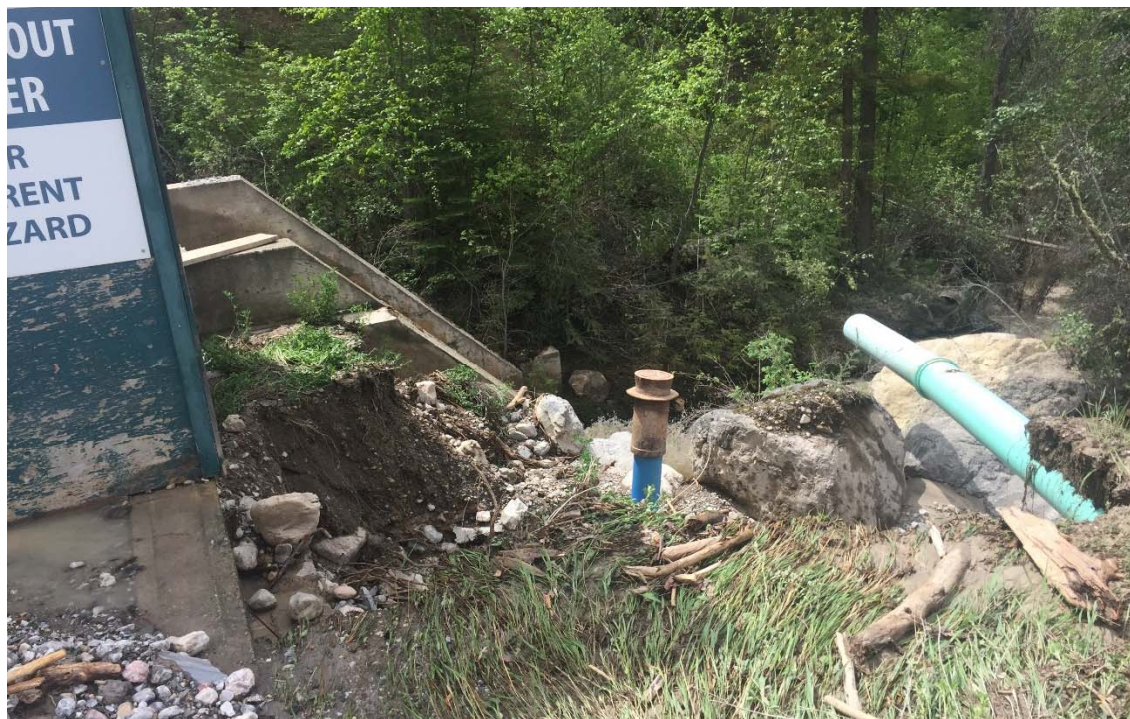
Photo 3: Erosion immediately downstream of the dam after the May 31 event. June 1, 2020.
