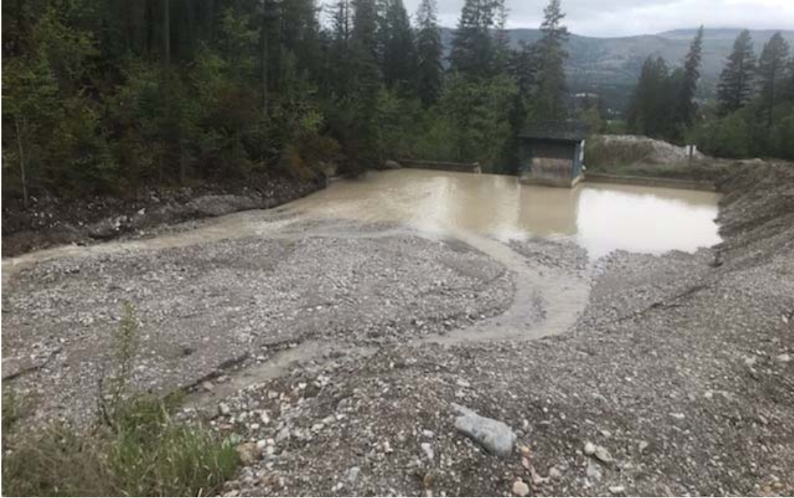
Photo 1: Cold Spring Creek Dam Reservoir partially filled with debris. May 22, 2020
