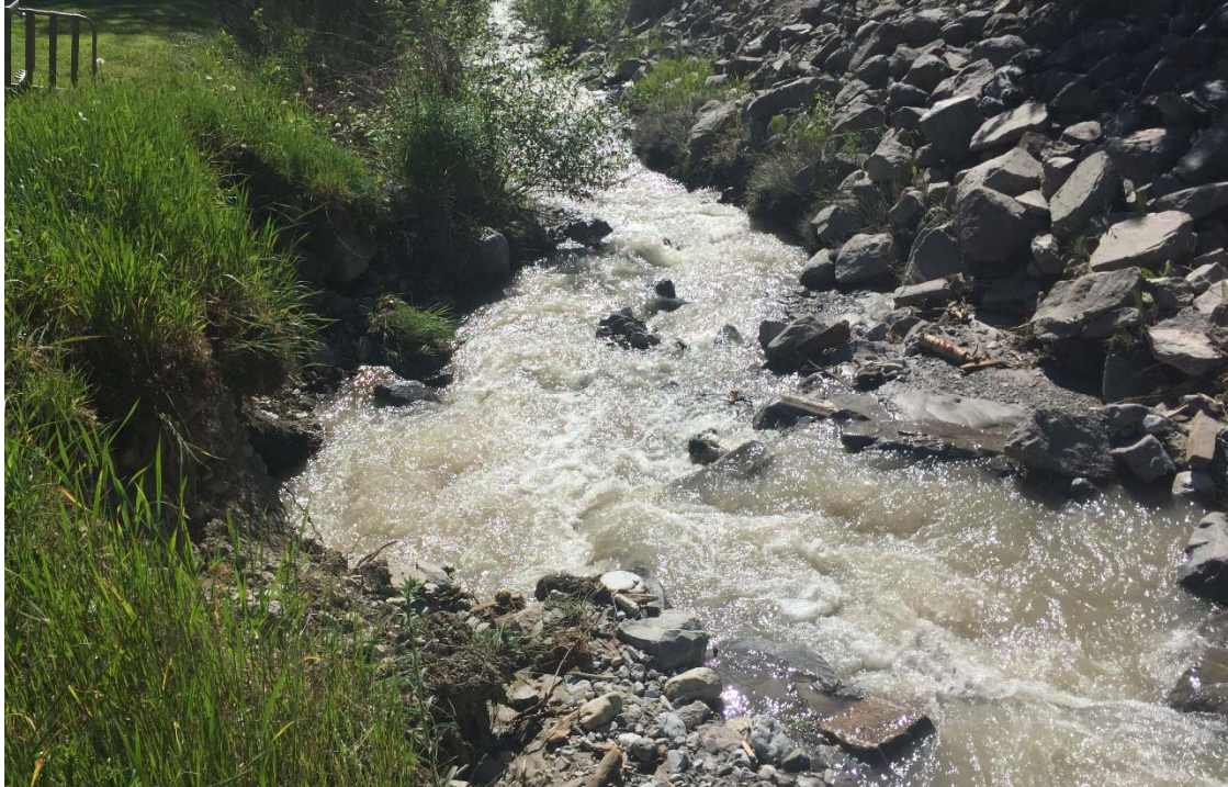
Photo 11: Bank erosion behind 2025 Riverview Road. June 3, 2020.
