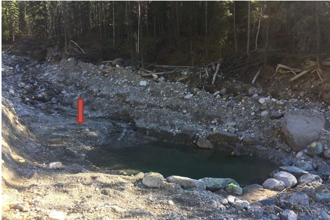
Photo 3: Weir 1 with debris flood material was removed. October 21, 2021.
