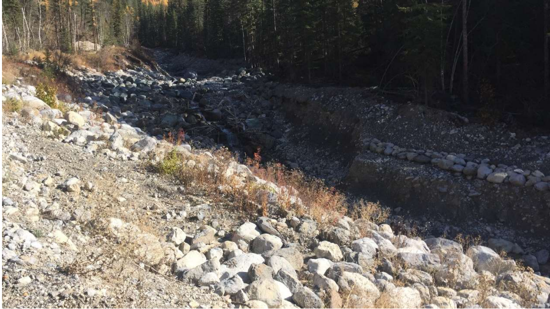
Photo 7: Weir 2 downstream face and scour that occurred primarily during the May 31 event. This was to be repaired in 2021 but was deferred due to the DFA funding not being approved. The armouring on the right bank was not damaged and the damage has not progressed significantly since the May 31, 2020 event. October 21, 2021.
