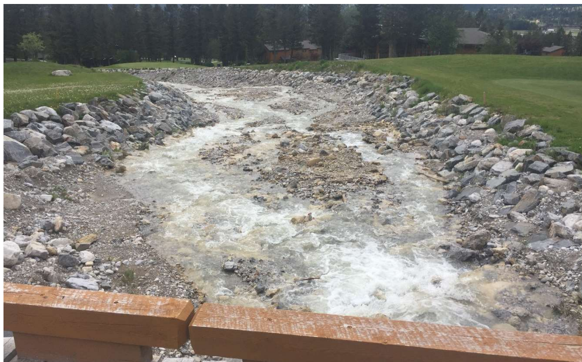
Photo 13: Golf course channel looking downstream from the cart path bridge on May 26, 2021. There was minimal debris deposition, flow was contained in the channel and the dikes were not impacted.
