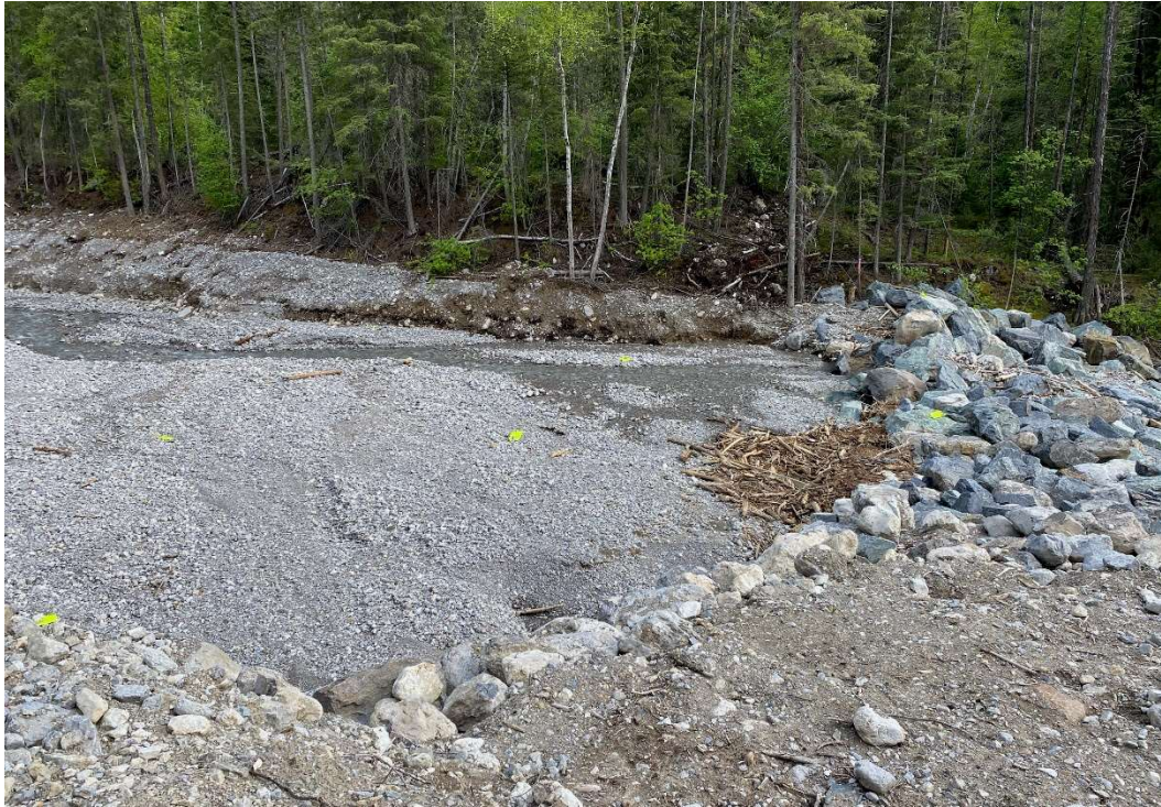
Photo 5: Weir 2 looking upstream. The basin is partially filled with debris flood material. May 29, 2021.
