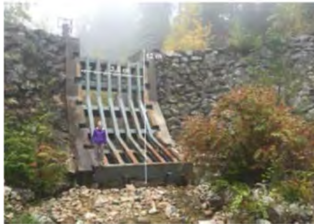
Figure 8. Example of proposed sloping outlet steel at McKay Creek East, District of North Vancouver (BGC and McElhanney 2022).
