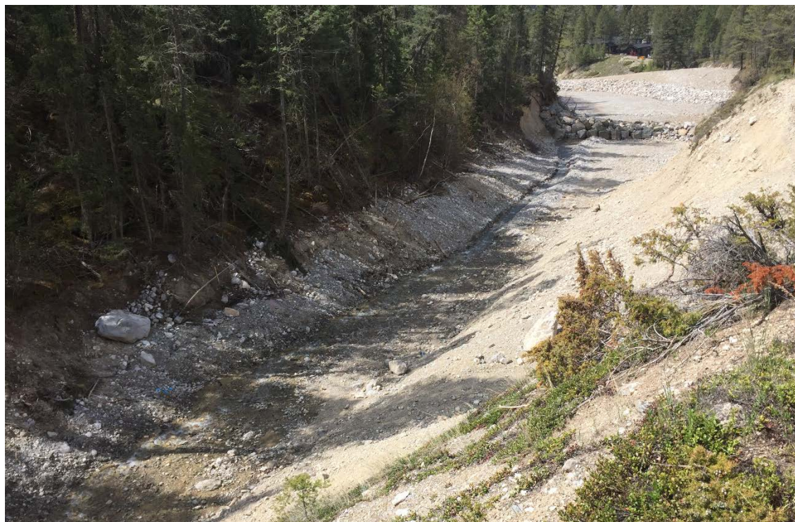
Photo 5: Weir #3 with bank armoring slightly past it.
