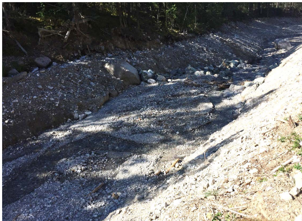
Photo 7: Weir #1, looking downstream. The storage area upstream of the weir was filled to capacity with approximately 1,225 cubic metres of debris flood material.
