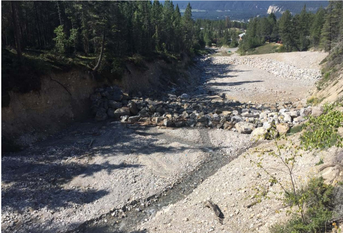
Photo 10: Weir #3, Looking downstream. There is a small amount of material deposited in front of the weir that came from the eroded channel upstream.
