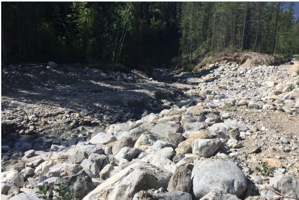
Photo 9: Bank protection downstream of Weir #2. Note the eroded channel below the protected bank. This material was transported downstream.
