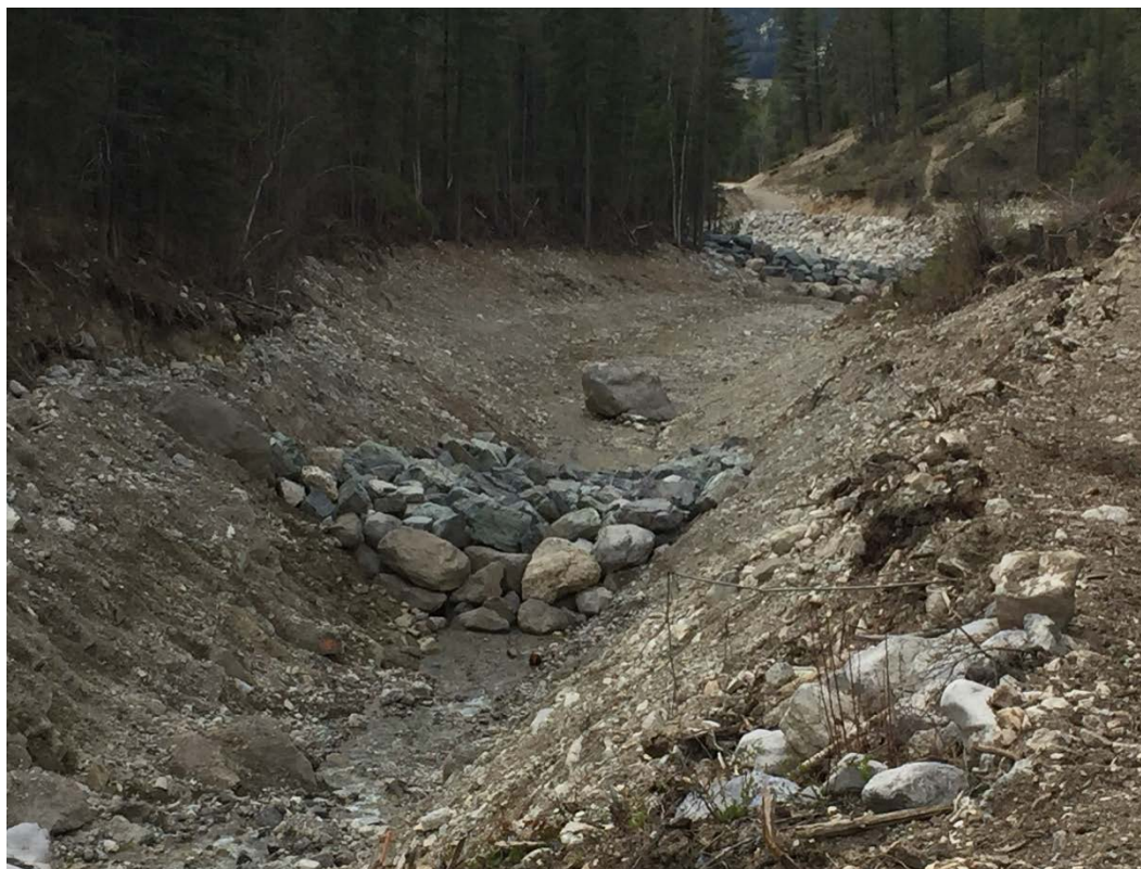
Photo 2: The uppermost weir in the system, Weir #1, is in the foreground; Weir #2 is seen in the background.
