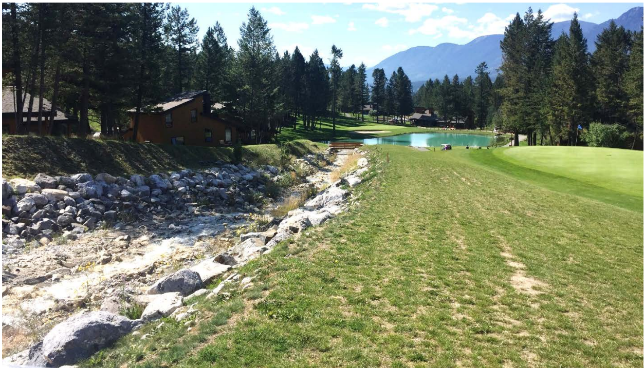
Photo 15: Looking downstream. The berms and bank protection on both sides are in good condition.
