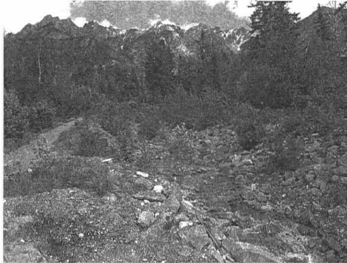
Cold Spring Creek, Site 3 – Vegetation growth within dike rip-rap 19/05/2005
