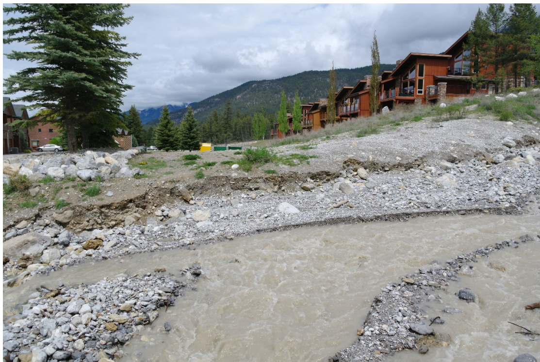
Photo 12: Upstream extent of the DFA works and bank protection. When comparing with Photo 7, the bank erosion, damage to the grade control structures and debris deposition is very apparent.
