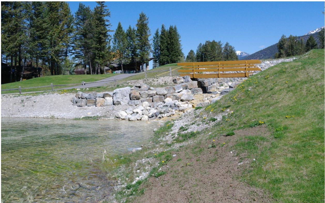
Photo 1: Downstream extent of the dike and bank protection works at the entrance to the debris pond.
