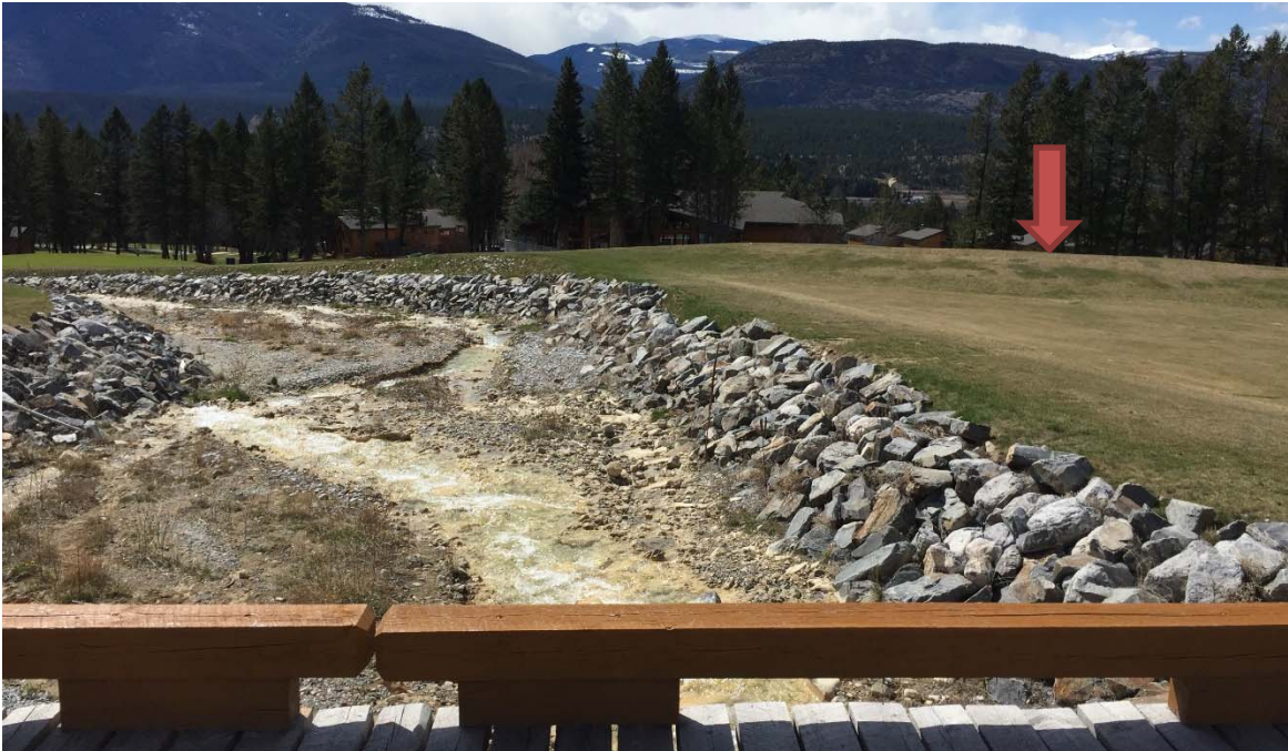
Photo 16: Golf course channel looking downstream from the cart path bridge. Channel is in good condition with some minor infilling from the August 2019 event. The dike on the right hand side of the channel (red arrow) is in good condition. April 23, 2020.
