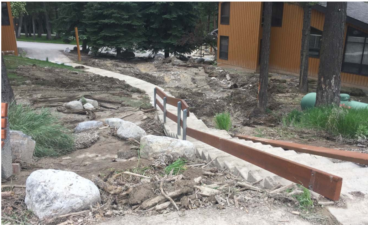
Photo 23: The flood flow exceeded the capacity of the spillway and the pond overtopped and water flowed between the condos on the downstream end of the pond. May 31, 2020.
