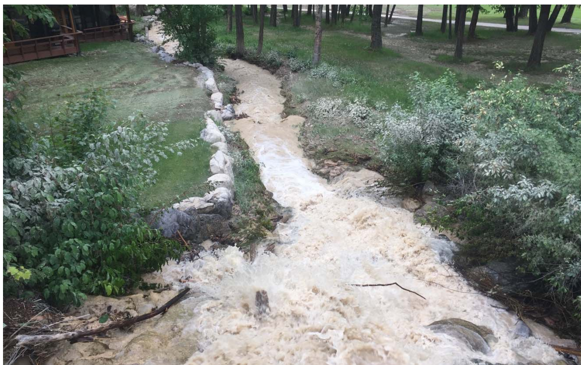
Photo 27: Pond outlet and channel during the May 31, 2020 event. The channel was not damaged and contained the flow. May 31, 2020.
