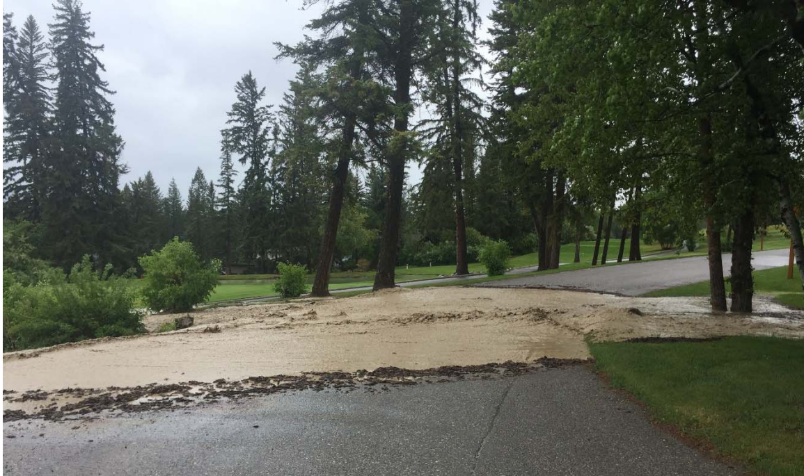
Photo 28: The culvert immediately downstream of the pond was blocked and could not contain the flood flow. Water flowed over the golf course and through residential properties before returning to the channel. May 31, 2020.
