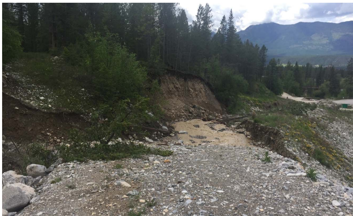
Photo 13: Erosion of the berm above the FHSR water mixing sheds. May 31, 2020.
