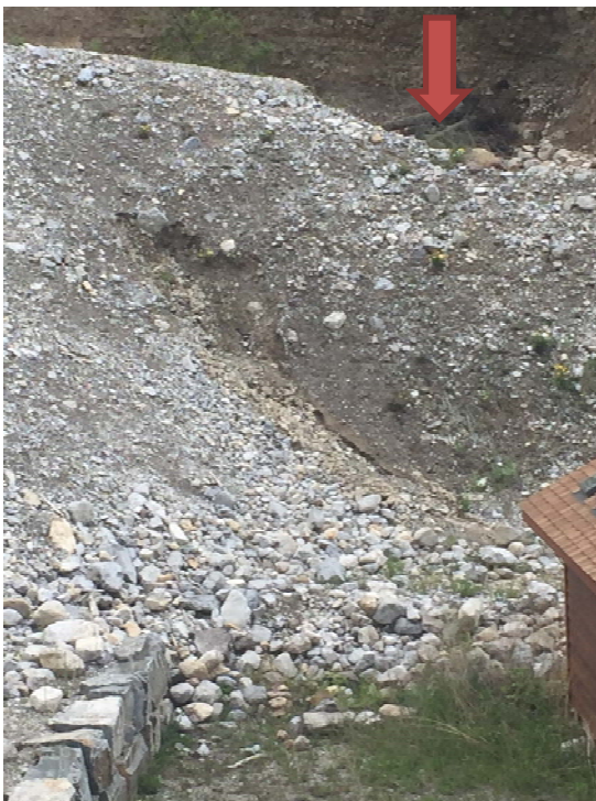
Photo 15: There was some minor seepage on the downstream face of the berm. Seepage was clear and stopped once the repair of the erosion was completed. The arrow shows the location of the erosion in the previous pictures. June 1, 2020.
