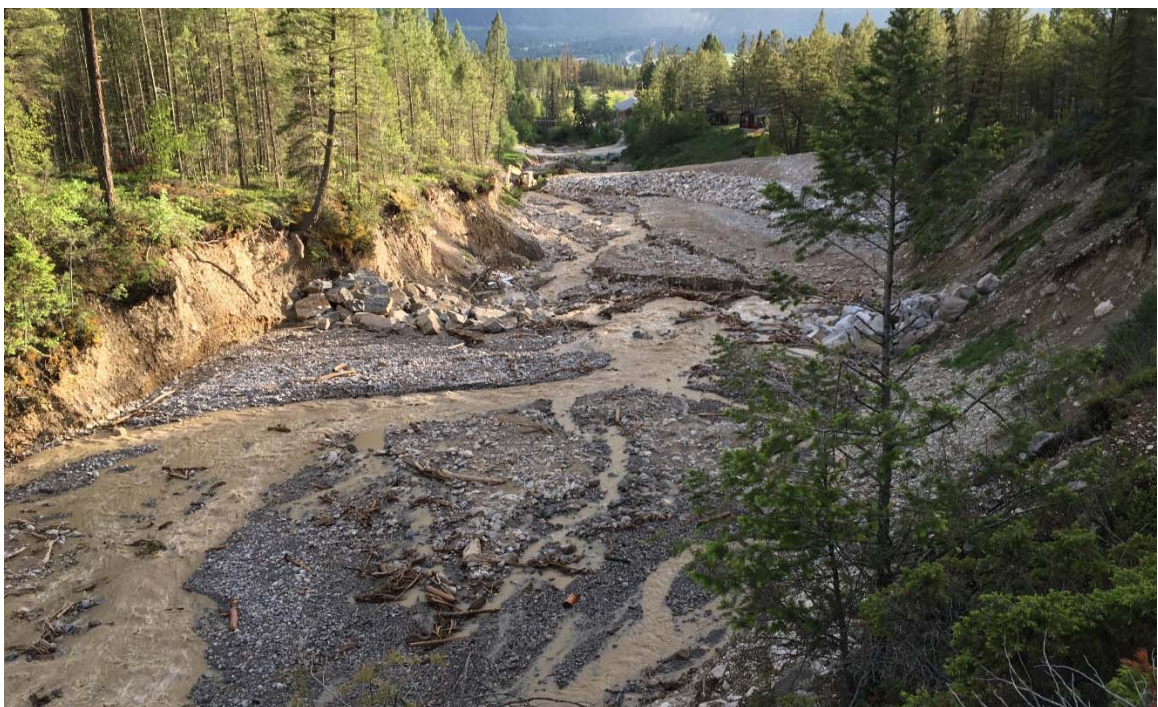
Photo 11: Weir 3 and basin after the May 31 event. There was minor scour downstream of the weir that did not require repairs. June 1, 2020.
