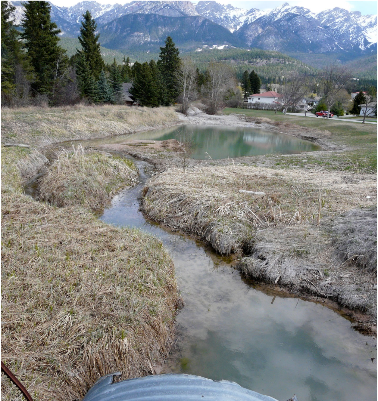
Photo 5: Cold Spring Creek outlet of debris trap showing siltation buildup up stream of the culvert
