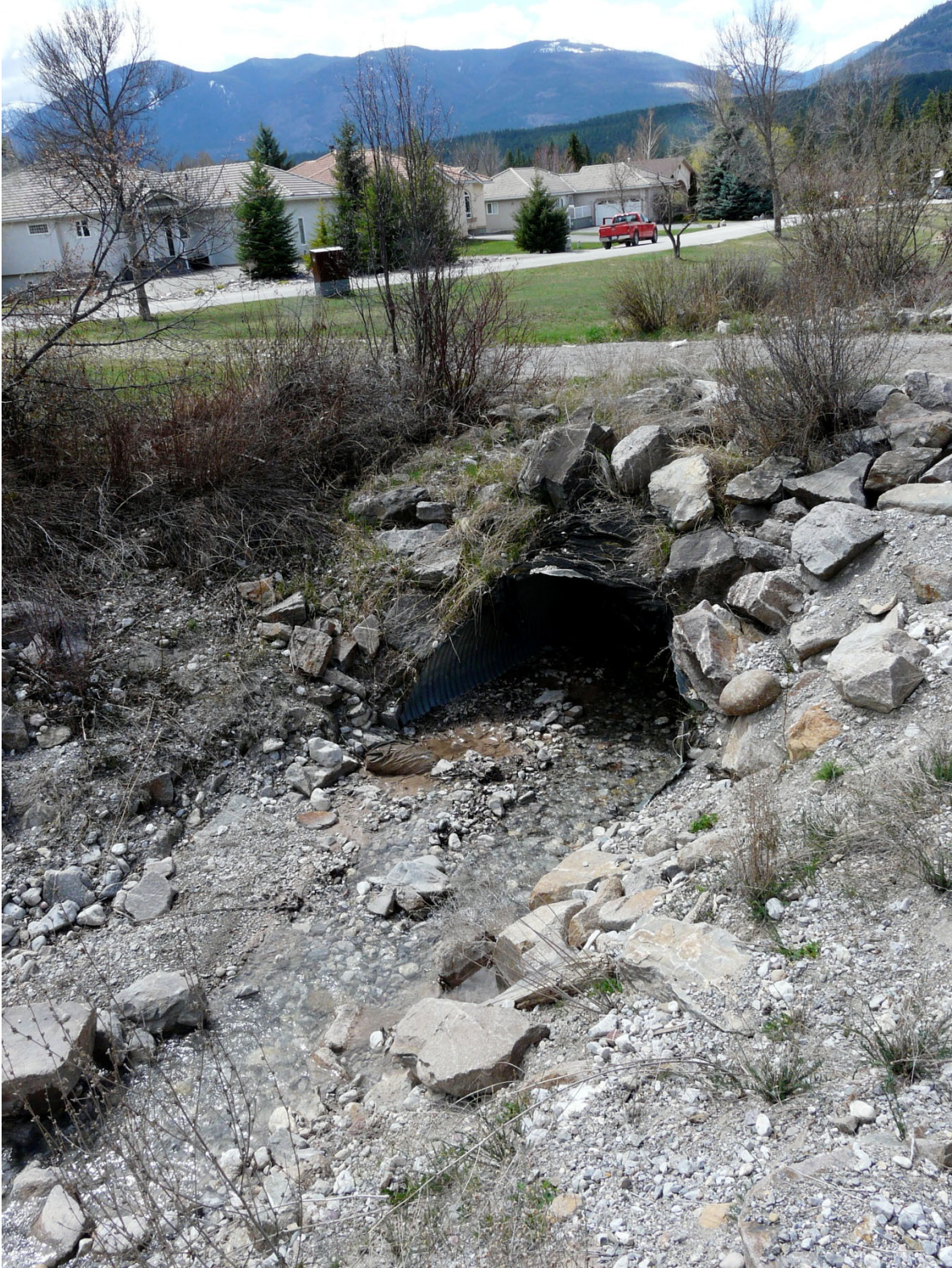
Photo 2: Lowest Cold Spring Creek Culvert Inlet with Sediment Build Up
