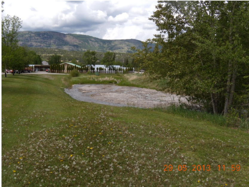
Debris Trap Sediment Deposition
