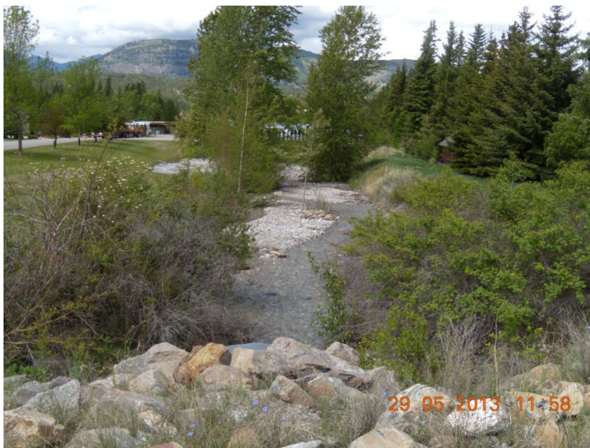
Debris Trap Sediment Migration into Cold Spring Creek Channel
