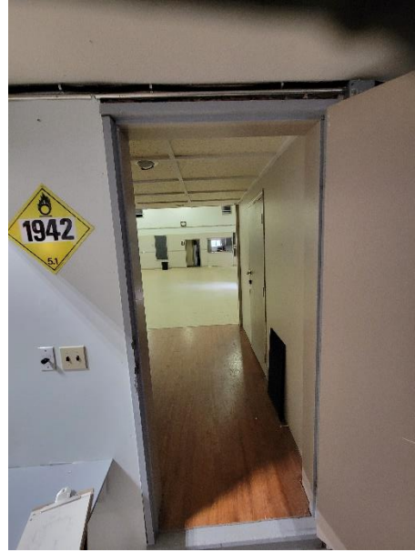
Photo 14 - Access door between fire hall and community hall is not fire rated
