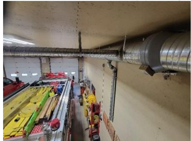
Photo 26 - Truck bay existing ventilation
