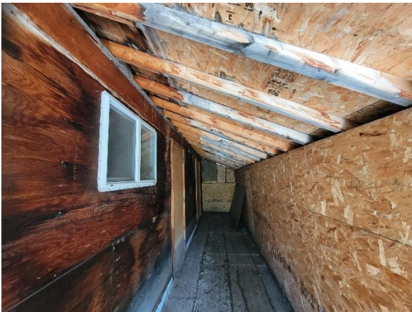
Photo 3 - South-eastern entry way over office/storage addition. Water damage to roof framing
