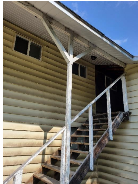
Photo 4 - South-eastern stairway roof beams, posts and guardrail require replacement.
