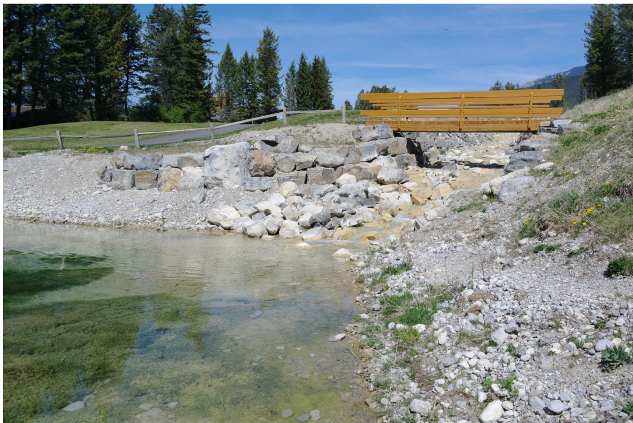
Photo 1: Downstream extent of the dike and bank protection works at the entrance to the debris pond.
