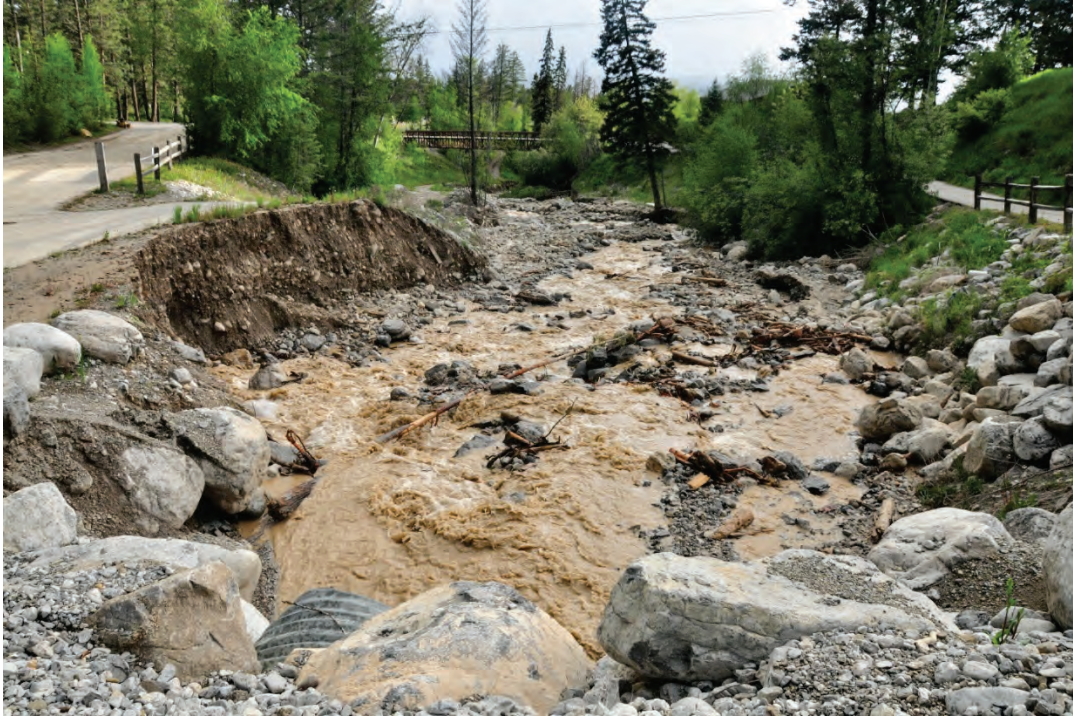
Photo 3.29 Bank erosion downstream of upstream most 4' culvert.
