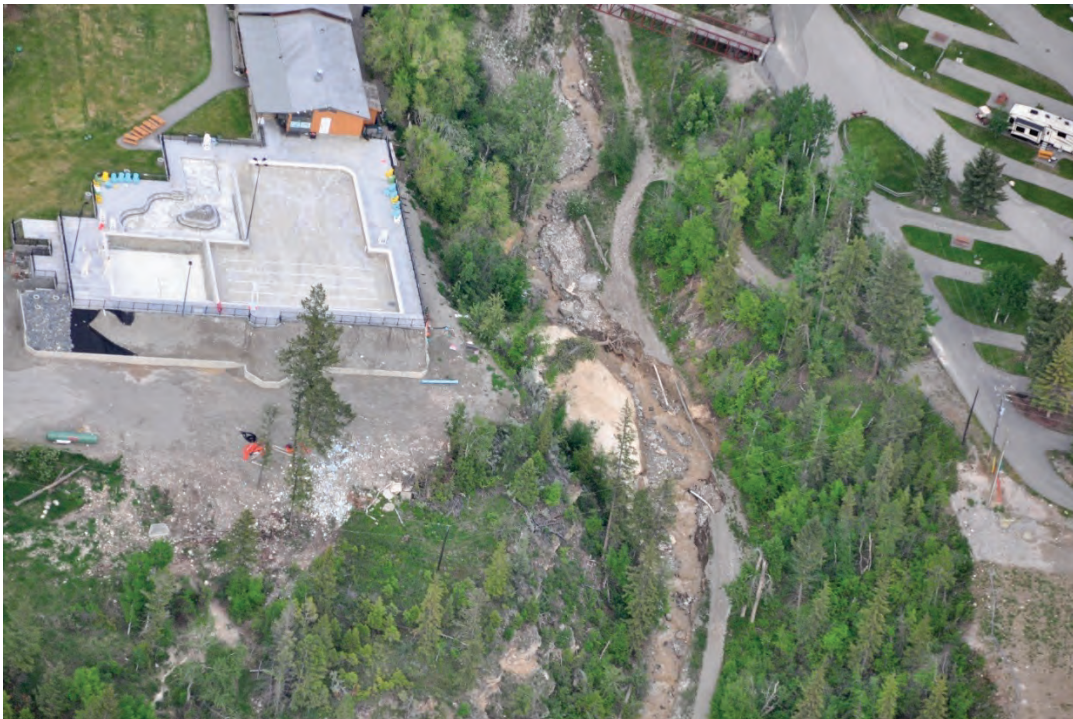
Photo 3.30 Fairmont Hot Springs pools and mineral rich water discharge point (light colored uniform textured deposit). Golf course irrigation pipe can be seen hanging in the air where the roadway has been eroded.
