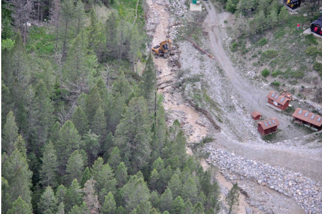
Photo 3.25 Bank erosion adjacent to hot springs intake huts immediately downstream of the downstream limit of the 2018 riprap placement as seen on the evening of June 1, 2020.
