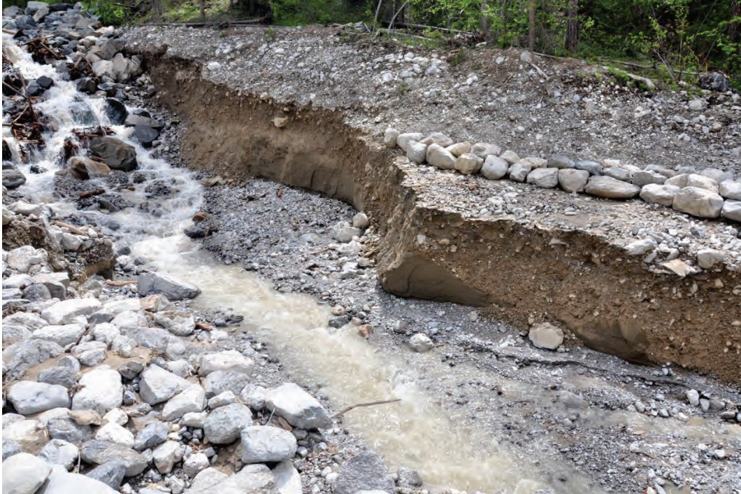
Photo 3.17 Incised stream channel at downstream limit of containment weir # 2. This section of channel needs grade control added and the banks protected to prevent additional channel migration and sediment removal.
