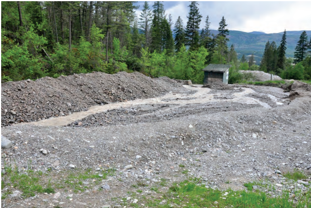
Photo 3.44 View looking downstream into dam headpond which has become filled with sediment. Note the presence of a abutment on river left at the crest of the dam but no evidence of a abutment on river right as the creek bed has aggraded and is above the abutment wall.
