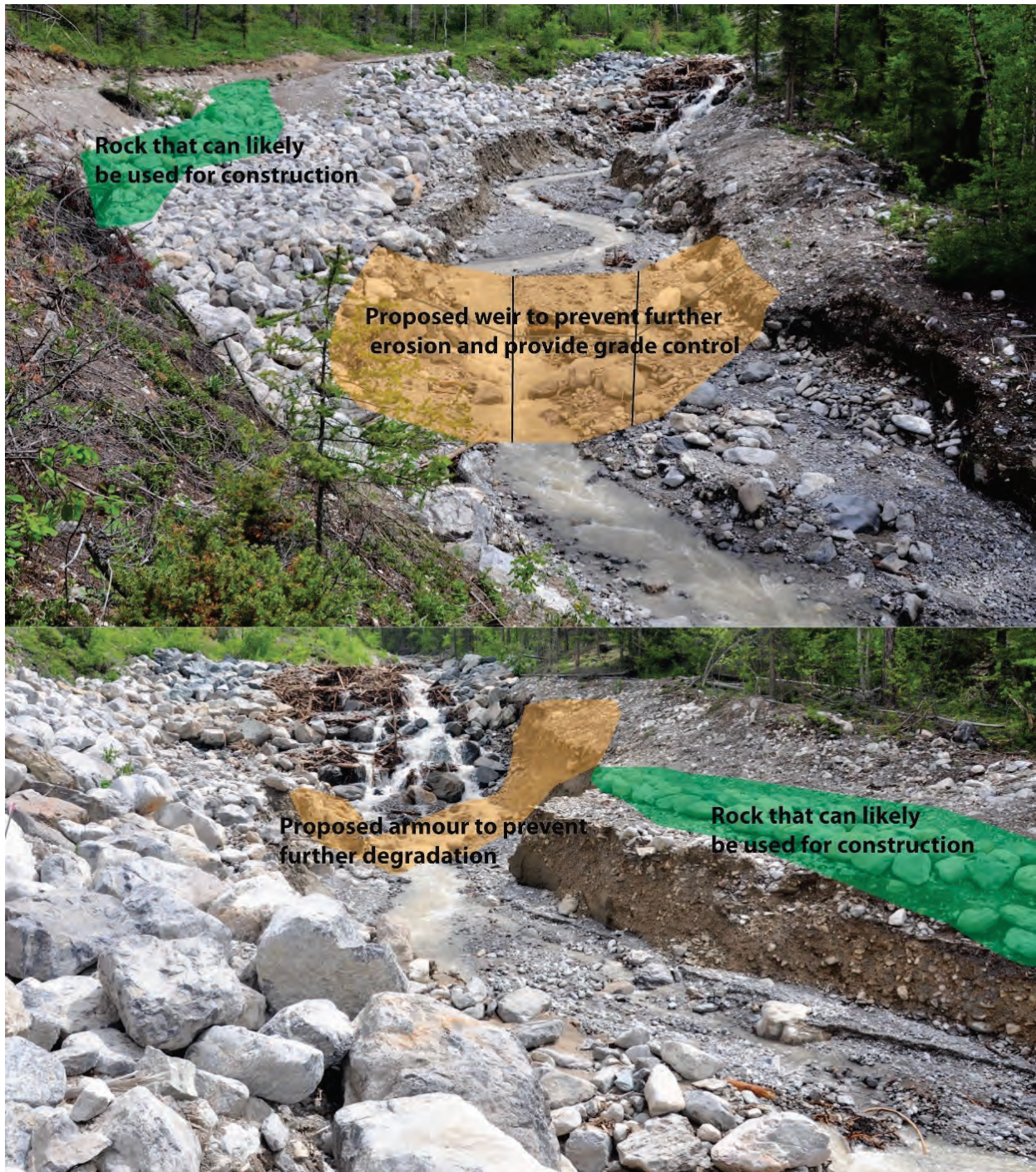
Figure 5.1 Proposed location of grade control repair using a rock weir; view upstream towards weir #2.
