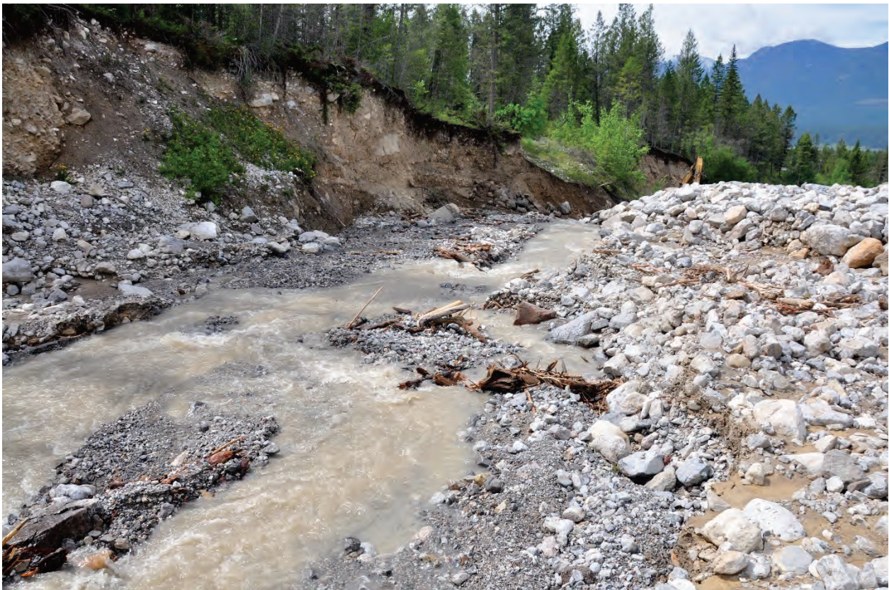
Photo 3.24 Degraded channel downstream of containment weir # 3 upstream of end of 2018 riprap placement. Hot spring intake buildings are over the berm to the right of the image.
