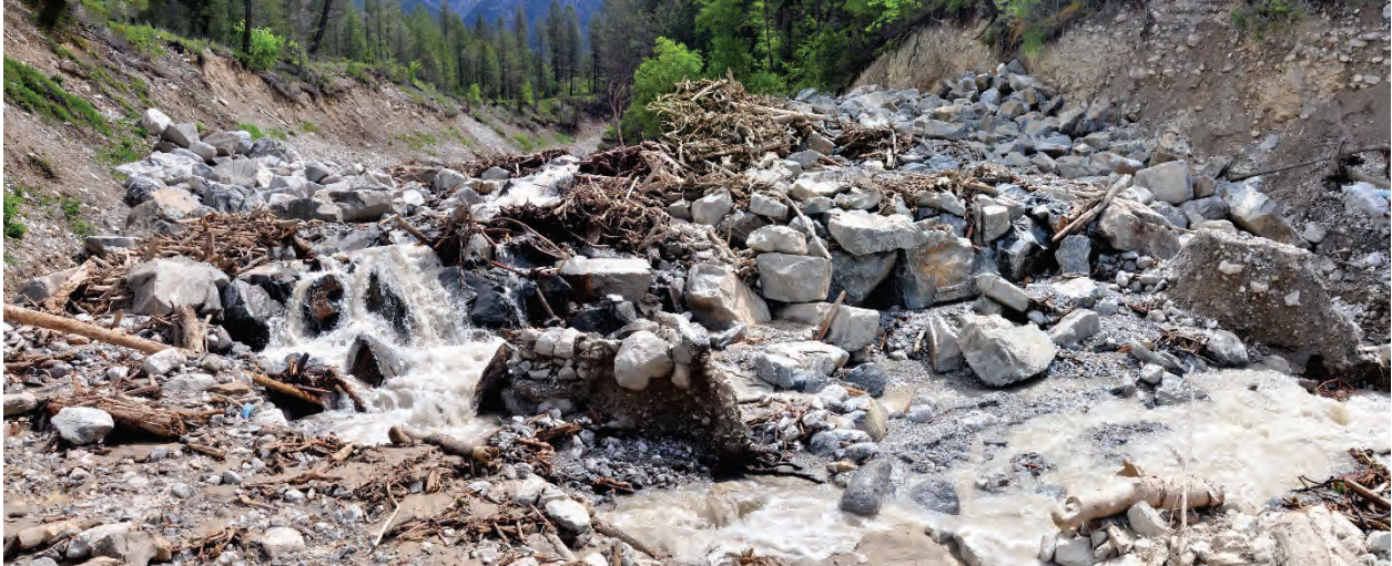
Photo 3.23 Downstream toe of containment weir # 3 showing limited scour after May 2020 event.
