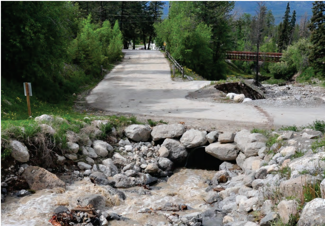
Photo 3.28 Four foot diameter culvert and road that was overtopped.
