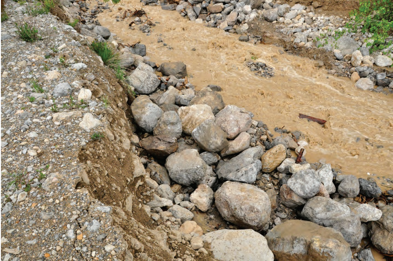
Photo 5.2 Section of berm upstream of first culvert along Fairmont Creek that experienced bank erosion and needs the bank protection rebuilt to prevent the creek from eroding through the berm and flowing down the hot spring intake access road.
