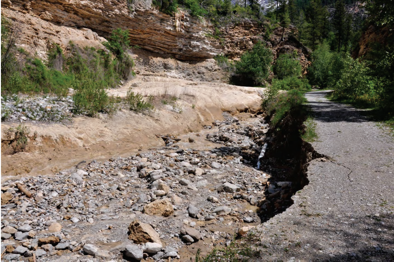
Photo 6.11 Limestone sediment accumulation on right bank (image left) of the creek and eroding bank on left bank of the creek with exposed irrigation water line.
