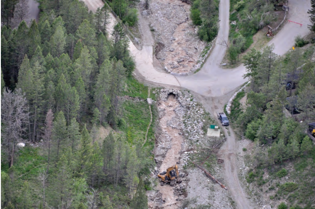
Photo 3.27 Upstream most 4' culvert viewed looking downstream. Creek overtopped road and debris line is visible crossing roadway on a diagonal.
