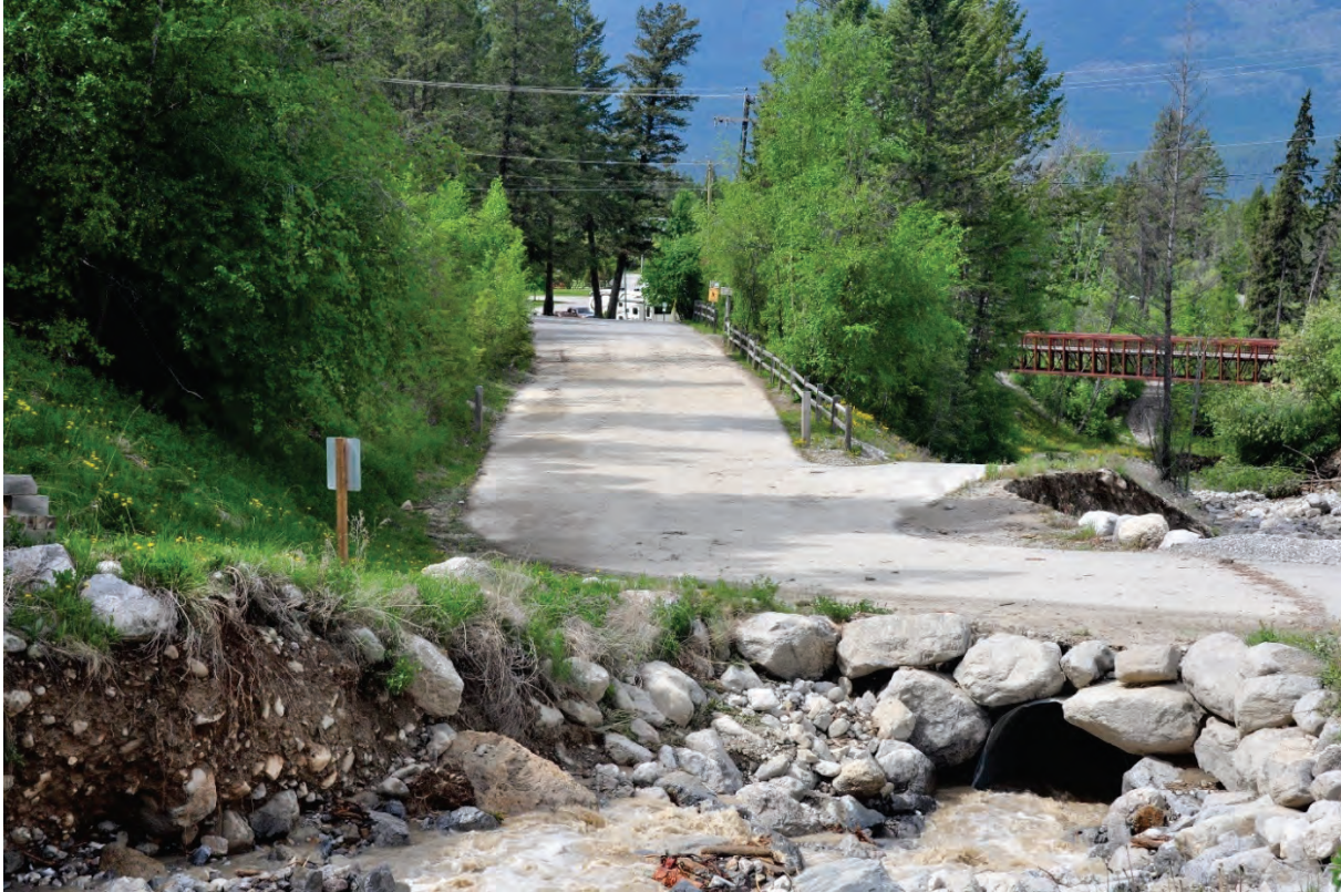
Photo 2.1 Upstream most 6' diameter culvert under Fairmont Resort Road that was overtopped and the downstream flooded area during the event. Debris line and mud covered pavement are visible in the photo.
