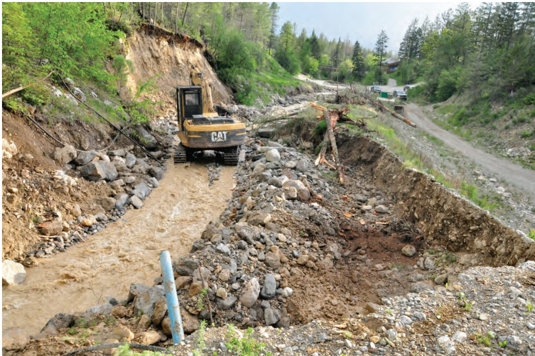
Photo 3.26 Evening of June 1, 2020 photo of eroded berm after initial re-alignment of channel by the excavator in the preceding hour. The small amount of remaining bank that separated the creek from the hot springs intake building is visible on image right and was about 1 m tall and 1.5 m wide.
