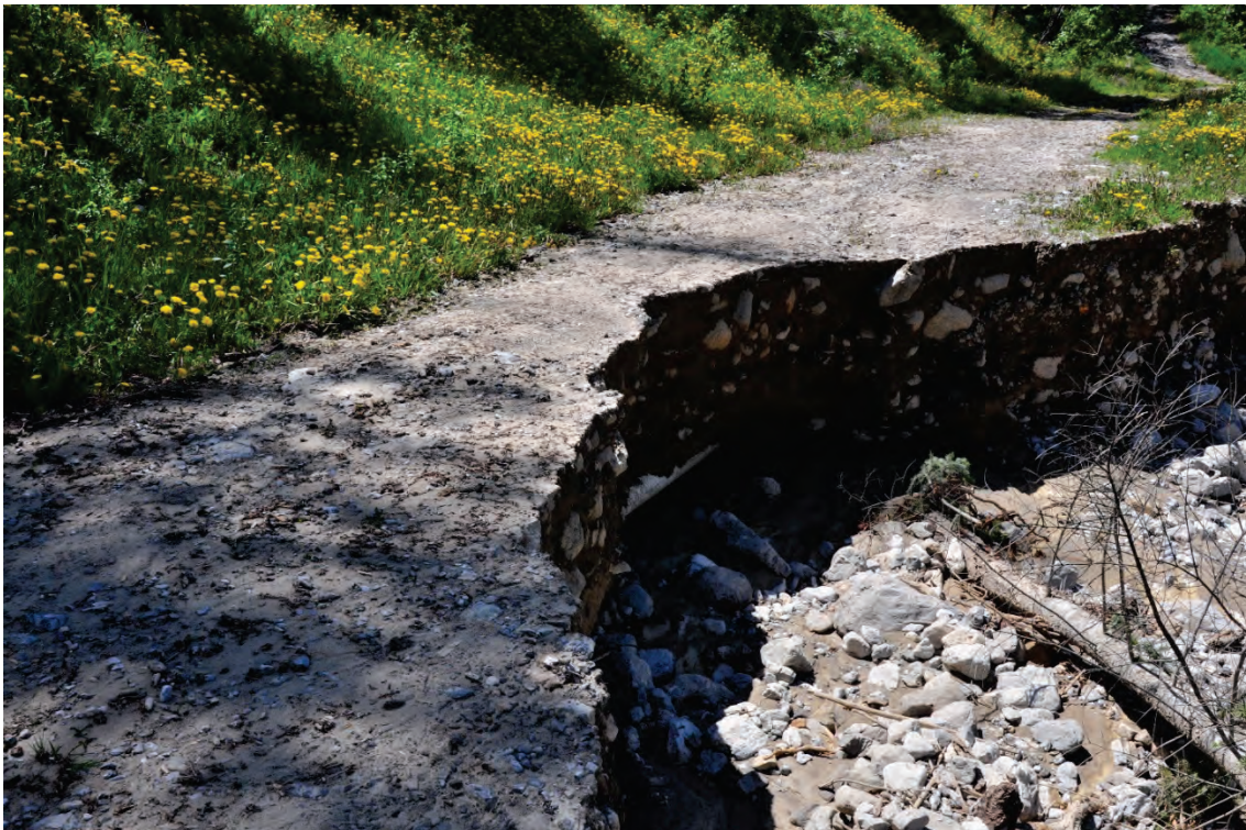
Photo 6.8 Section of access road that was washed out and exposed irrigation waterline.
