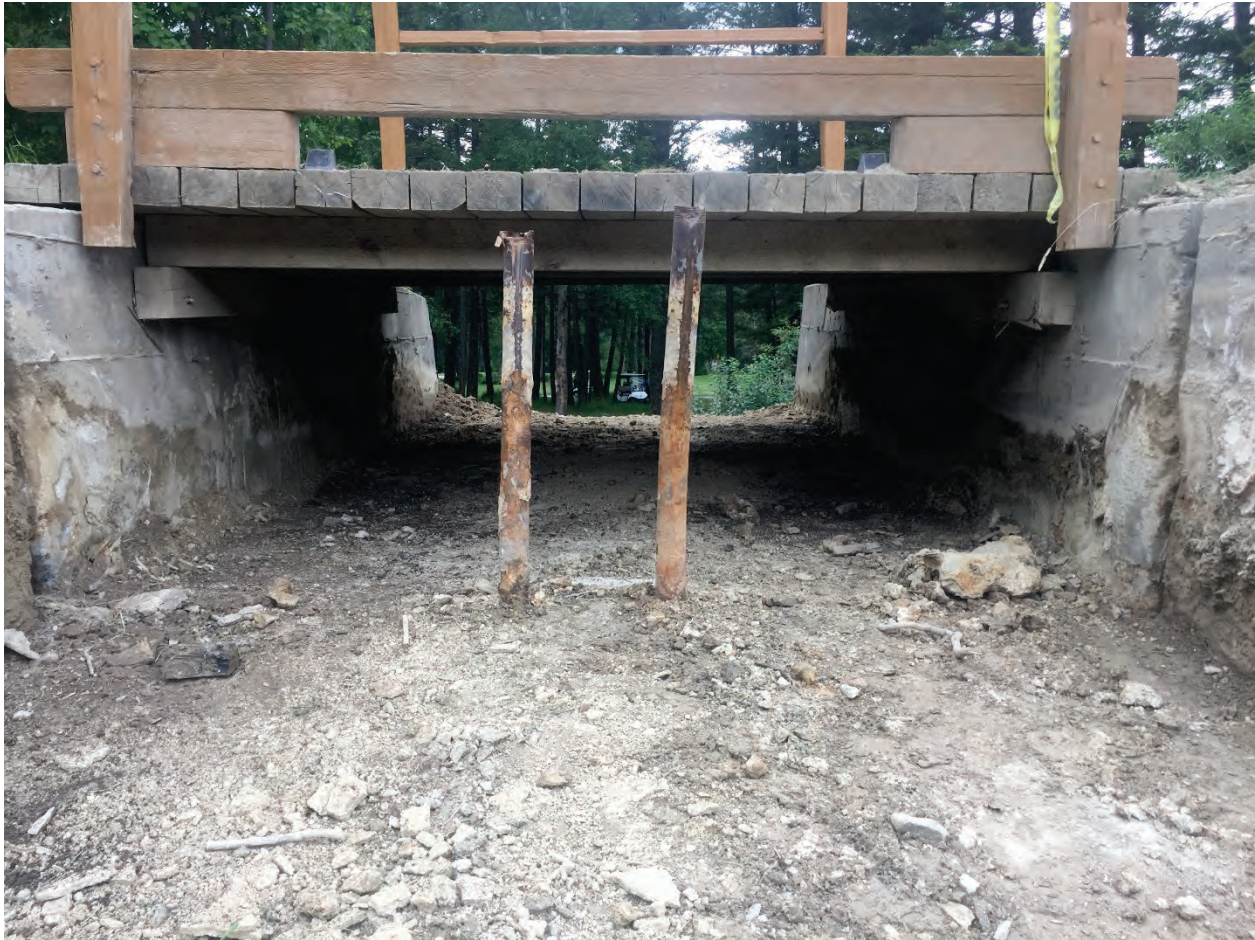
Photo 6.5 Channel draining golf course pond after accumulated sediment had been removed by contractor. Photo by Kara Zandbergen.
