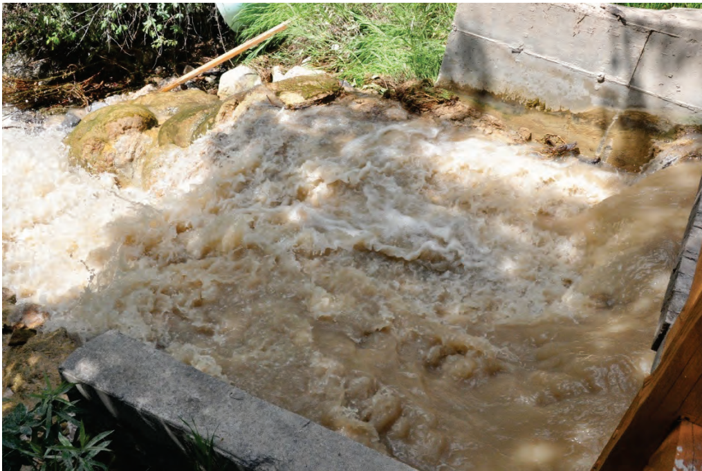
Photo 6.2 Current outlet of golf course pond and 4 meter tall cascading channel that leads into Fairmont Creek. It appears that a sill is currently blocking water passage below the boardwalk on the right side of the image.
