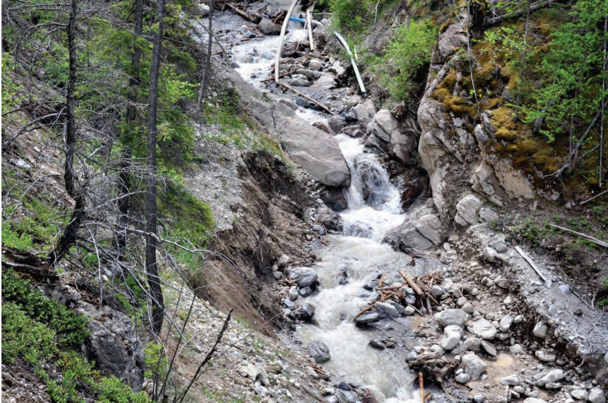
Photo 3.19 Bedrock constricted and bedrock grade controlled portion of Fairmont Creek between weir # 2 and weir # 3. Small slope failures from most recent event are visible, as well as perched terraces from 2012 event.
