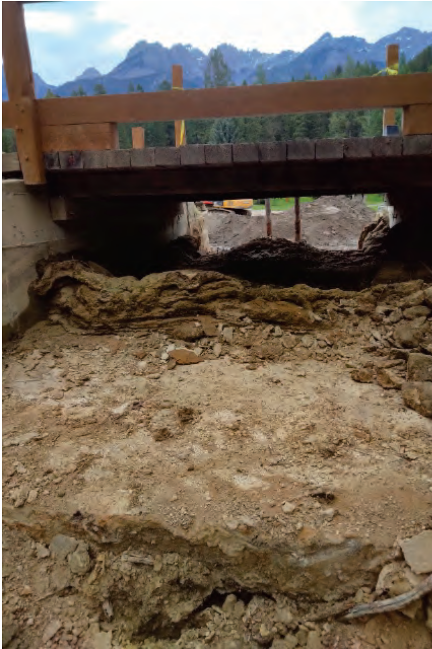
Photo 6.3 Downstream end of channel at pond outlet following flood event. Photo provided by contractor removing sediment from pond.
