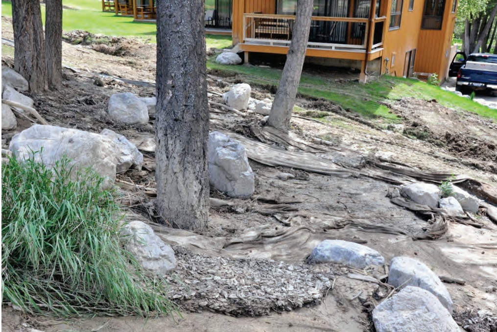
Photo 6.1 Eroded soils downslope from golf cart road that was overtopped when water levels in the golf course pond sediment trap were raised.
