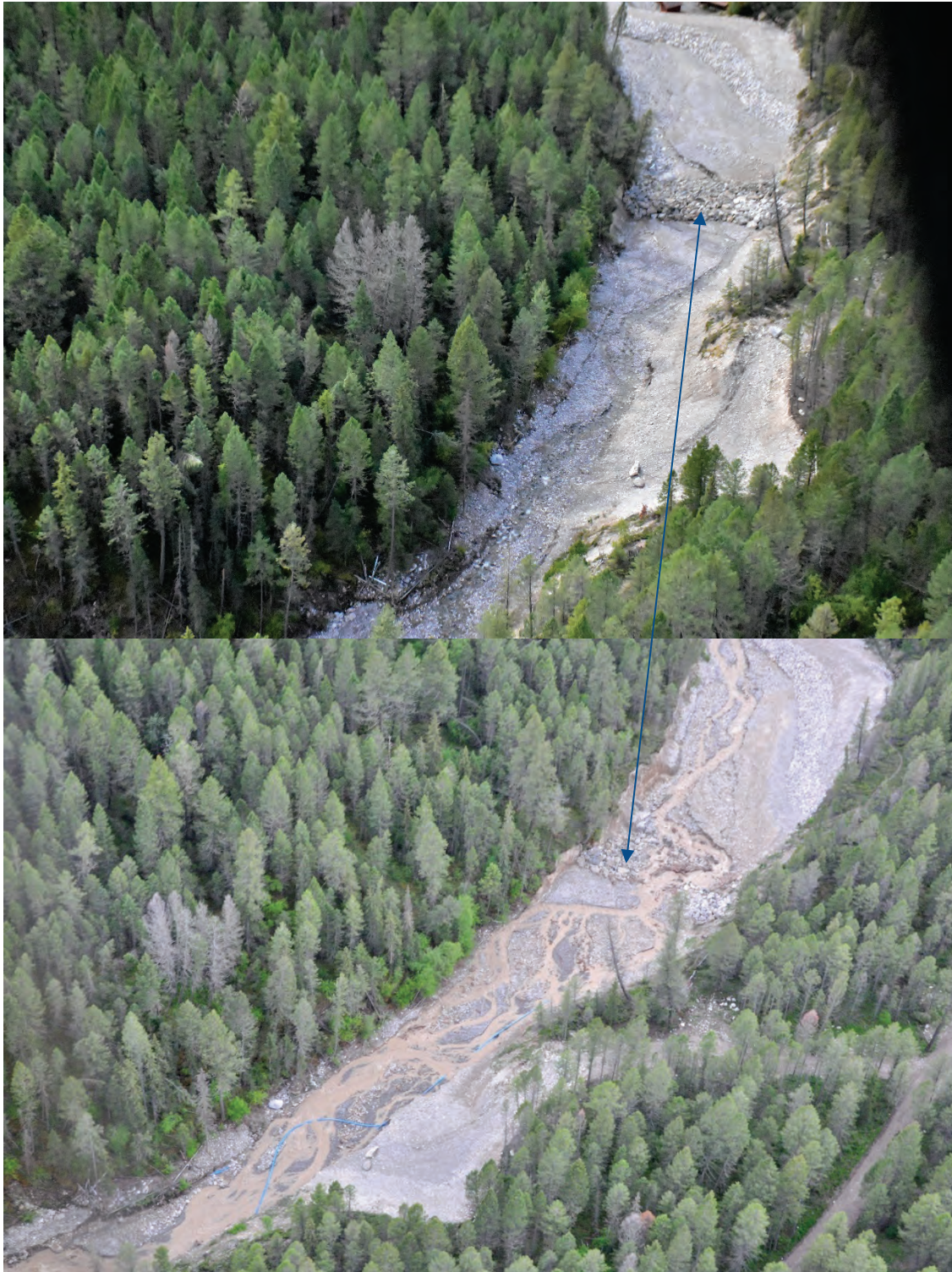
Photo 3.20 Sediment containment weir # 3 on September 17 2019 (top) and June 1 2020 (bottom). Flow from bottom of image to the top. Blue pipe is located in area where sediment accumulated upstream of weir.
