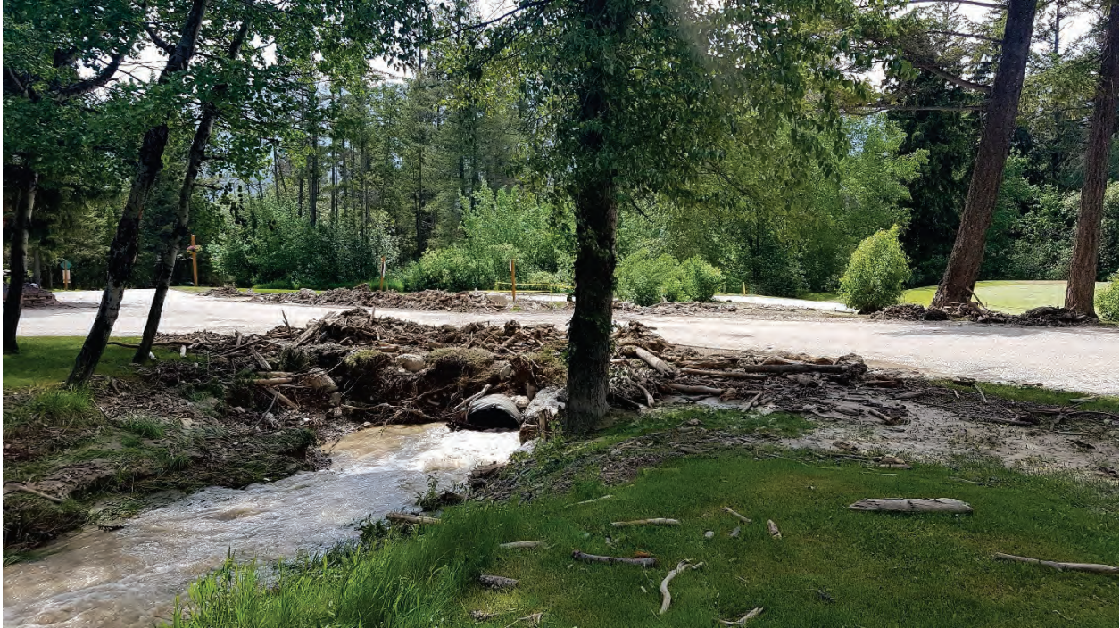
Photo 3.32 Culvert that was overwhelmed during the flood event that is located 250 m downstream of the golf course pond on road providing access to Fairmont Mountainside Vacation Villas.
