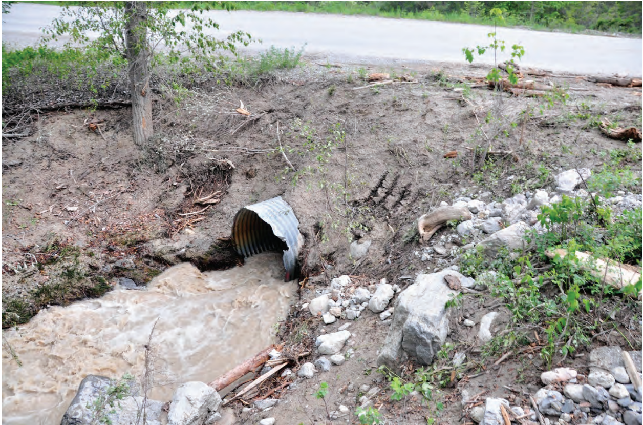
Photo 3.45 Cold Spring Creek crossing under Fairmont Resort Road downstream of Fairmont Resort dam.
