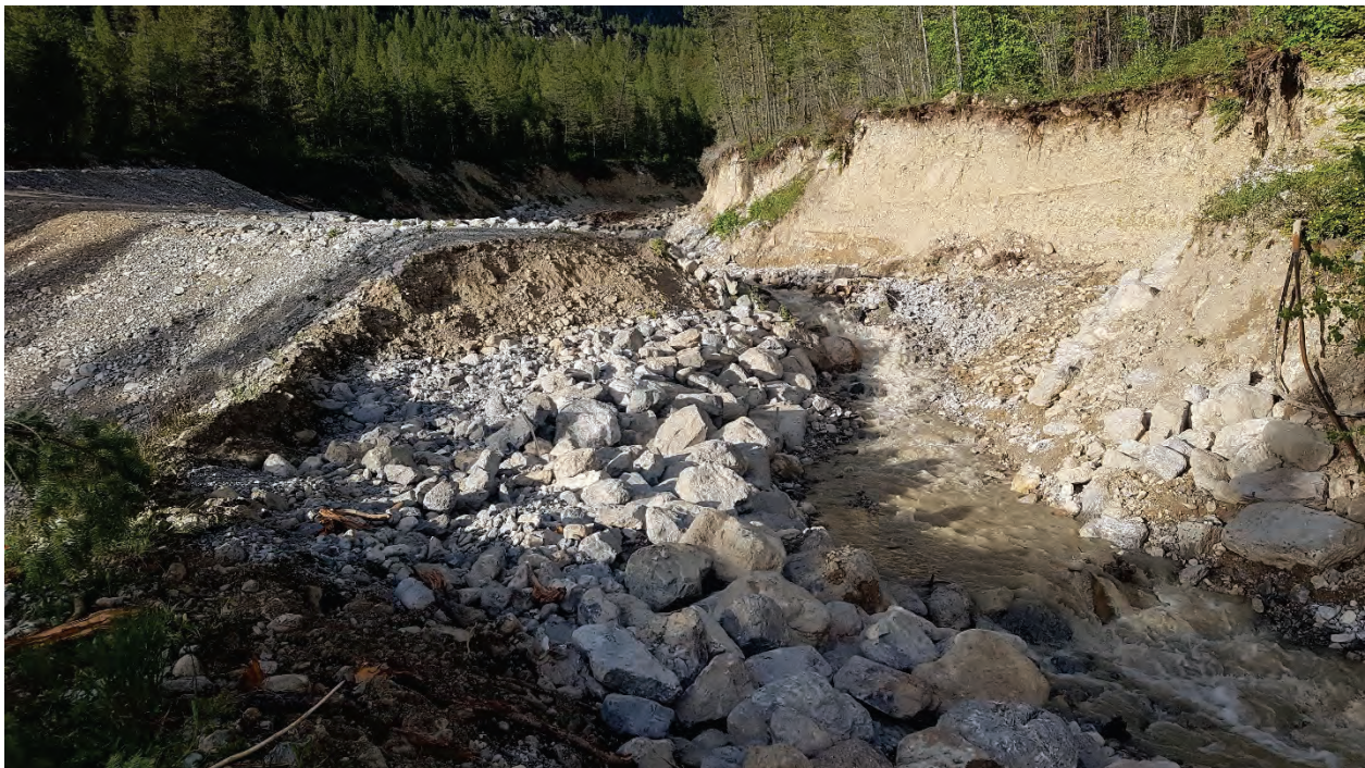
Photo 5.1 Partially repaired channel adjacent to hot spring intake on evening of June 2 2020.
