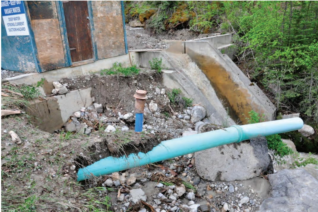
Photo 3.43 Downstream face of dam showing path of water to right side of spillway and resulting scour.
