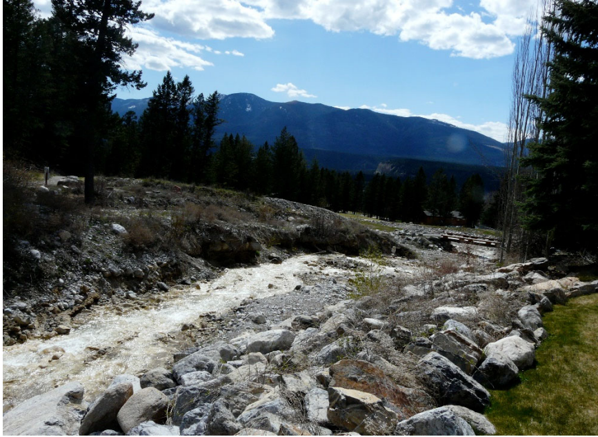
Photo 12: Left Bank Scour Locations Along Lower Area of Marble Canyon Section
