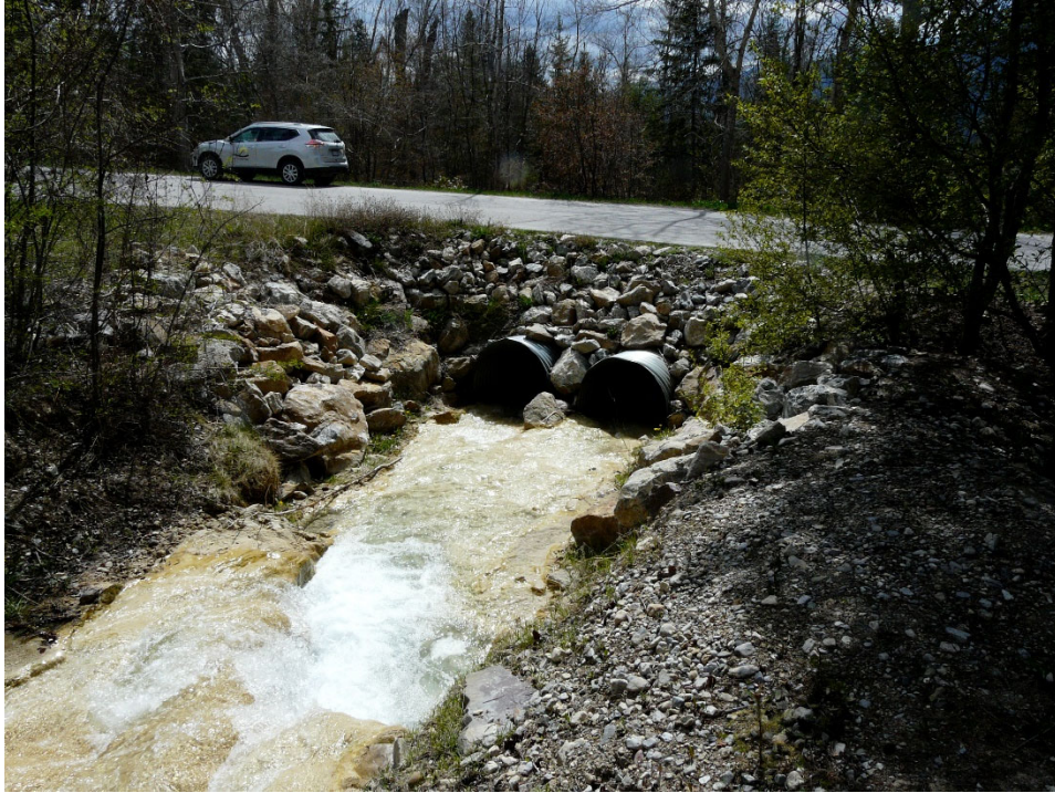
Photo 18: MoTI Culvert Infilling, Last Culvert Along Fairmont Creek Before the Columbia River
