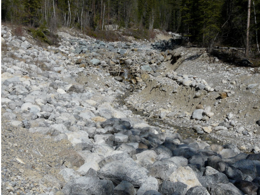
Photo 8: Woody debris on DS Slope of Weir 2, Left bank scour
