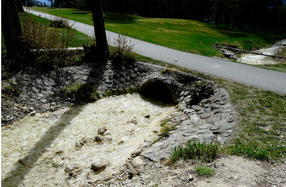
Photo 17: Second Culvert Downstream of Hole 12 Debris Trap/Pond, Inlet Obstruction Present FHSR Culvert
