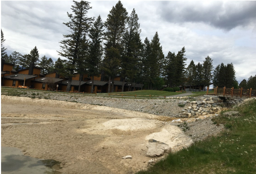
Photo 15b: Hole 12 Pond With Underflow Discharge in Effect. Sediment Build Up Very Evident on Left Side of Pond Inlet
