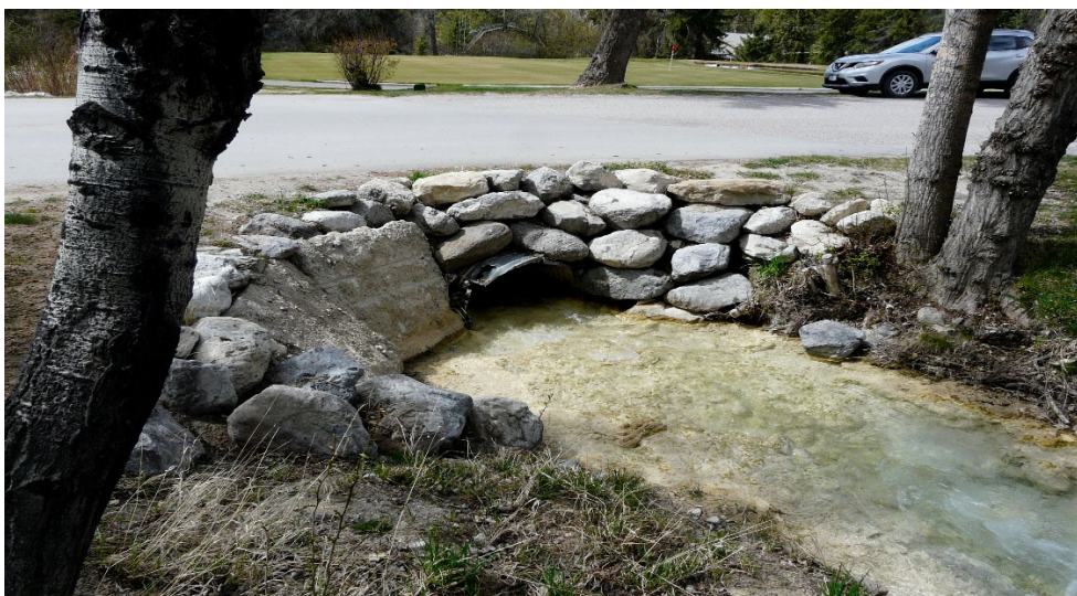
Photo 16: First Culvert DS of Hole 12 Debris Trap/Pond Outlet, Inlet Obstruction Present FHSR Culvert
