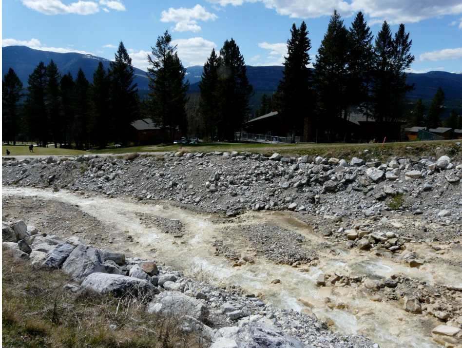
Photo 14: Exposed Bank Protection at Bend on Fairmont Creek Above Hole 12 Debris Trap
