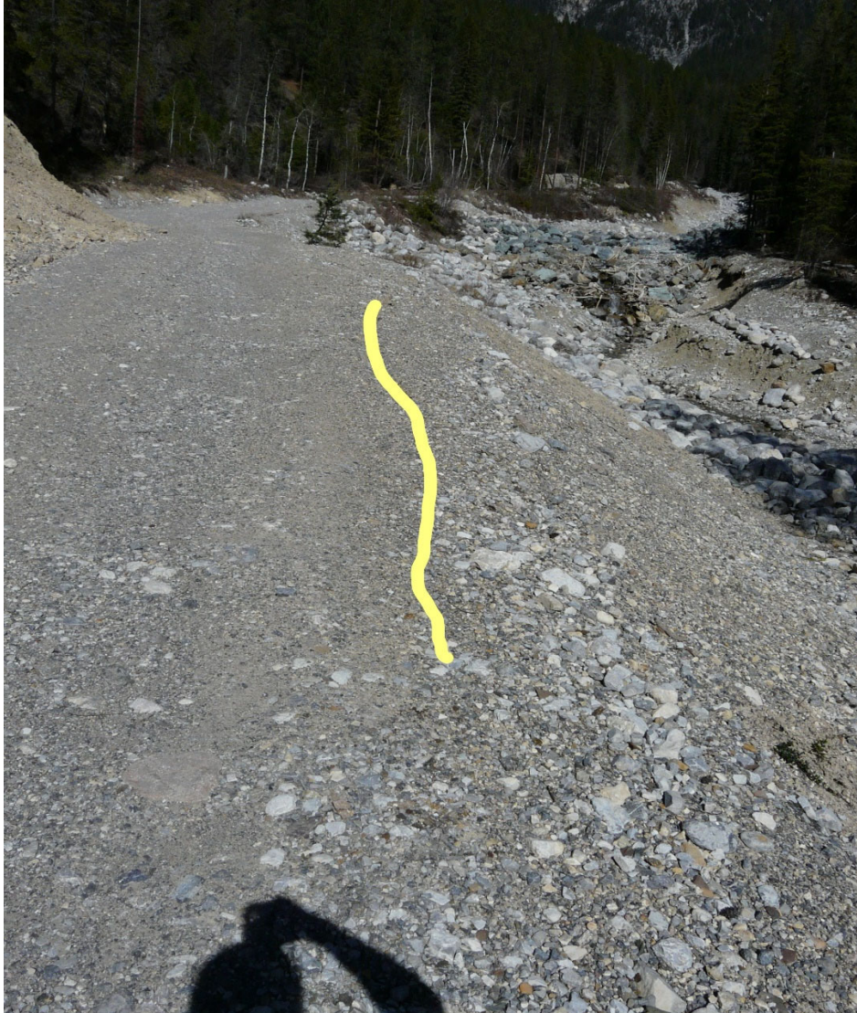
Photo 11: Tension Crack on Fairmont Creek Debris Trap Access Road
