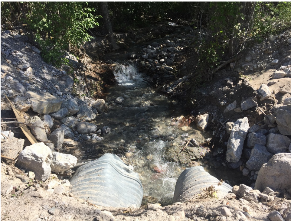
Photo 7: Culvert at the crossing of Hot Springs Road looking upstream. The culverts were plugged and debris was removed as an emergency measure to restore flow.
