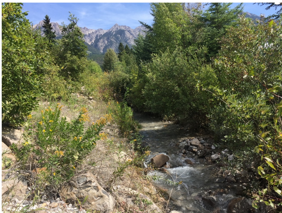
Photo 11: Facing upstream from the culvert in Photo 9. Vegetation management is required and will be completed in 2020.
