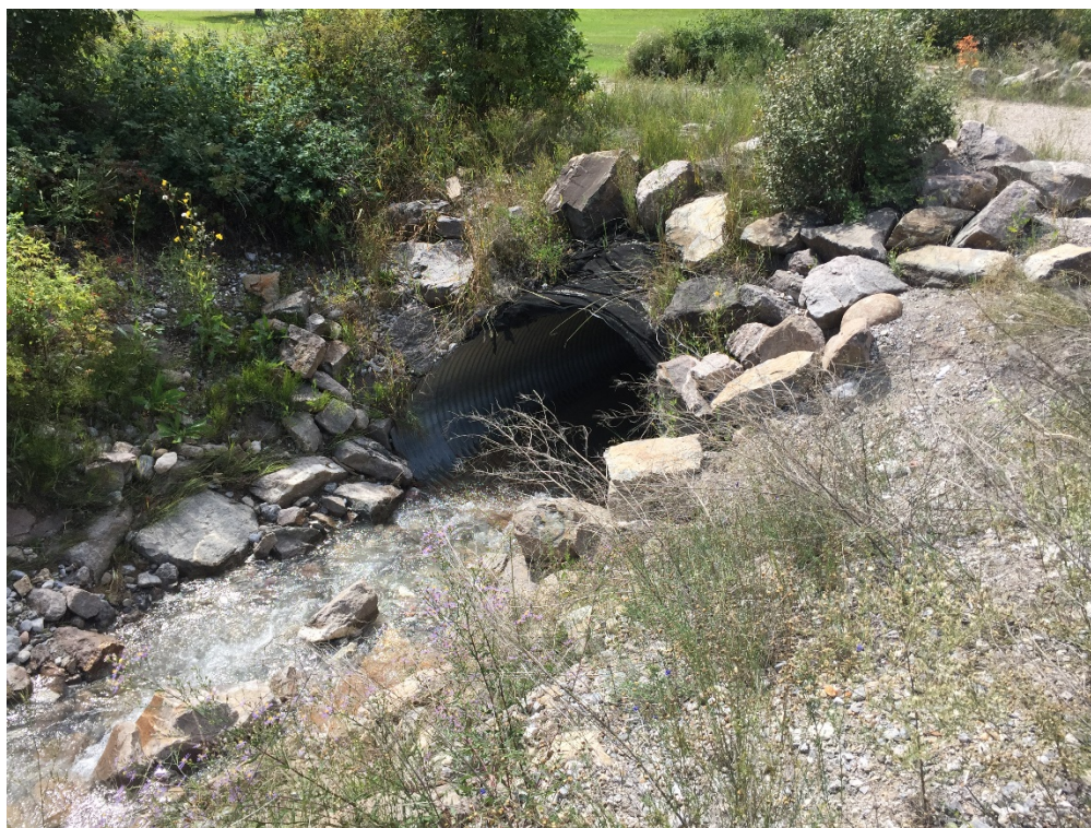
Photo 9: Culvert just upstream of the lower debris trap. The culvert is in good condition with very minor piping that is being monitored.
