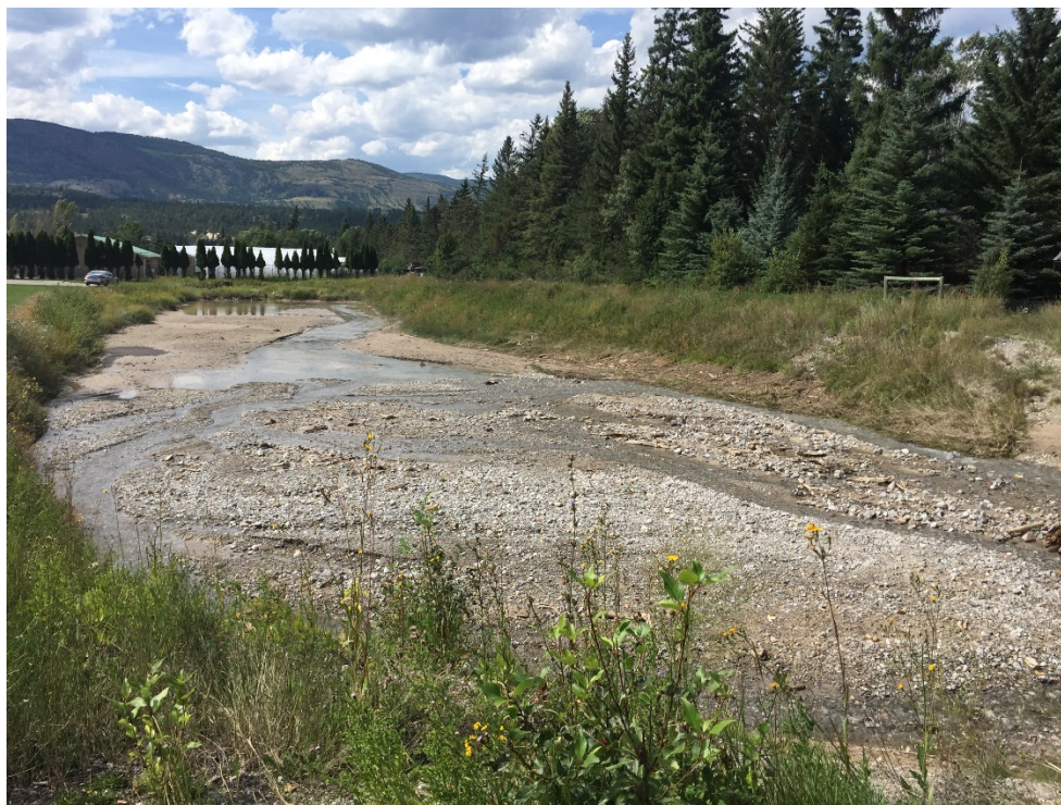
Photo 8: Cold Spring Creek lower debris trap.
