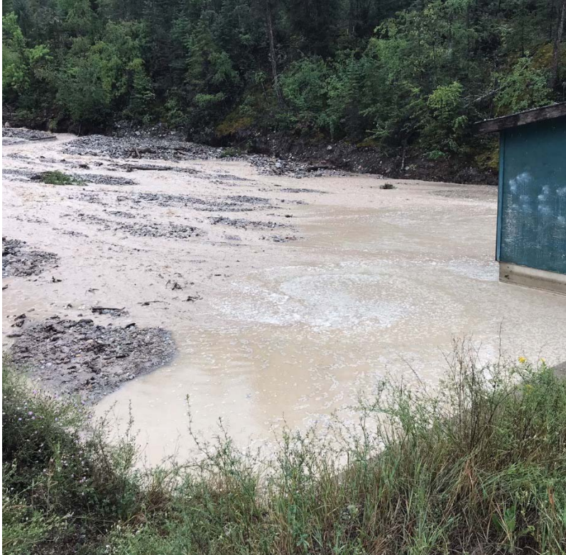
Photo 4: Cold Spring Creek Dam reservoir immediately after the August 12, 2019 event.
