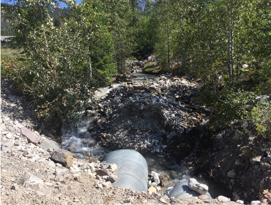
Photo 6: Culvert at the crossing of Fairway Dr looking upstream. The culvert was plugged and debris was removed as an emergency measure to restore flow.
